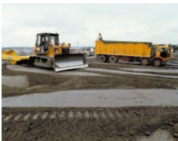
PFA compaction during construction of the A52 trunk road. Photo courtesy of UK QAA
