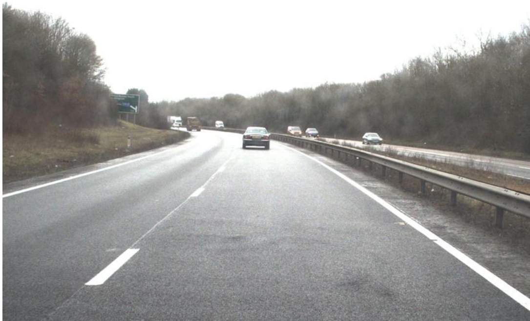
Figure 14 Area of roughness that was not present before resurfacing
