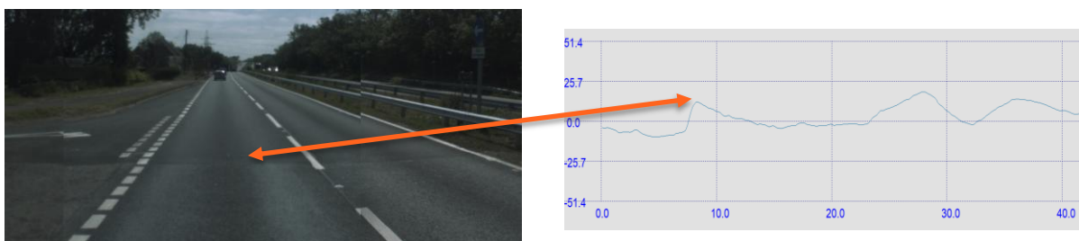
Figure 5 Unevenness at the transition joint at the start of a site
