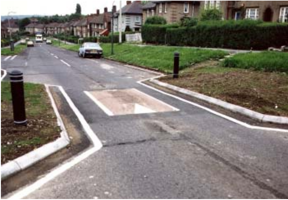
(a) Single cushion layout - buildouts from both sides — Lindsay Avenue (site 28) (Picture TRL)
