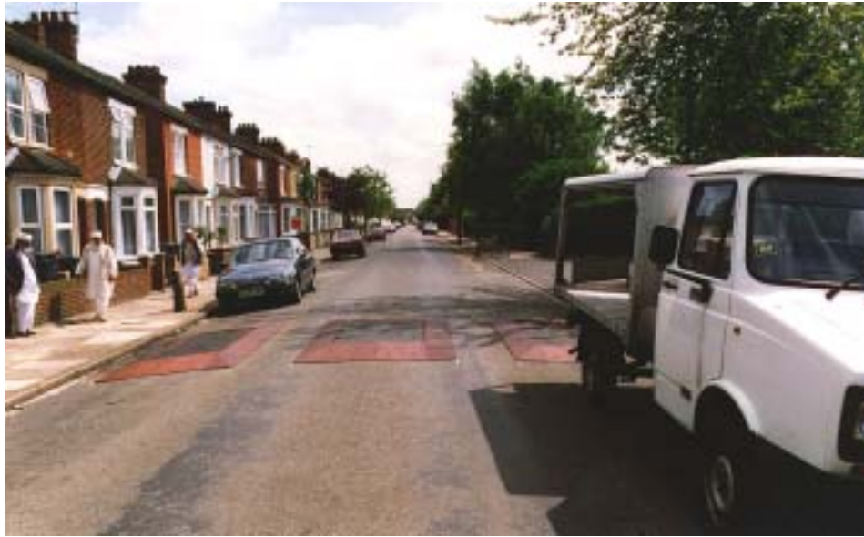
(a) Residential street with three-abreast cushions of composite construction — Coventry Road (site 1) (Picture courtesy of Bedfordshire CC)
