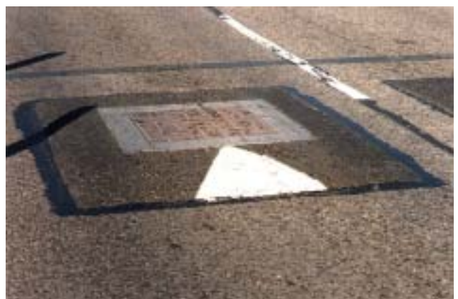
(f) Composite, block paving/asphalt Windmill Road (site 8) (Picture courtesy of Hertfordshire CC)
