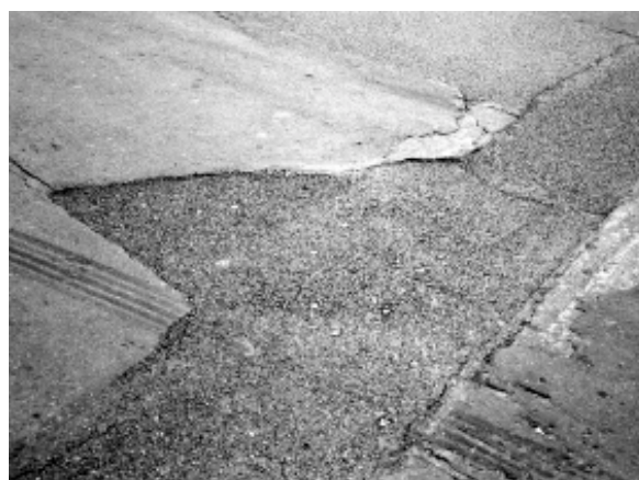
Plate 16 Poor quality final reinstatement
