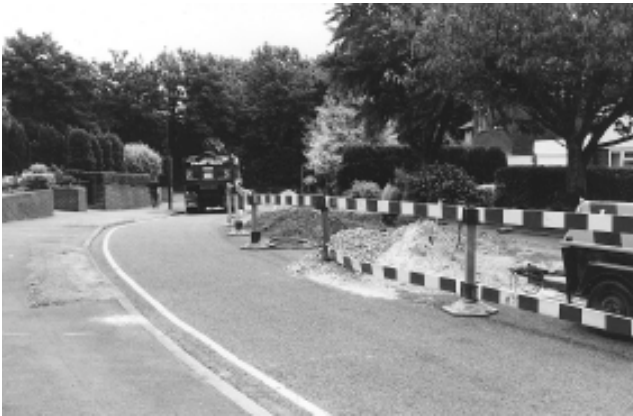
Plate 1 Poor material stockpile storage
