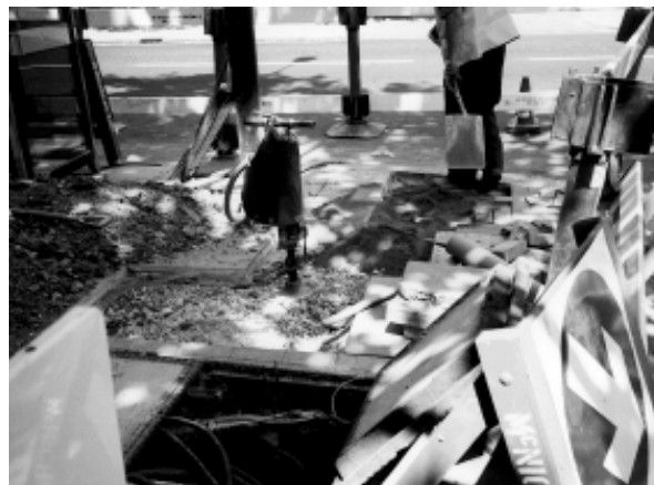
Plate 15 Untidy working practice, unsuitable compaction plant
