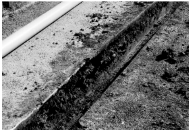
Plate 5 Undercutting increases the risk of poor compaction
