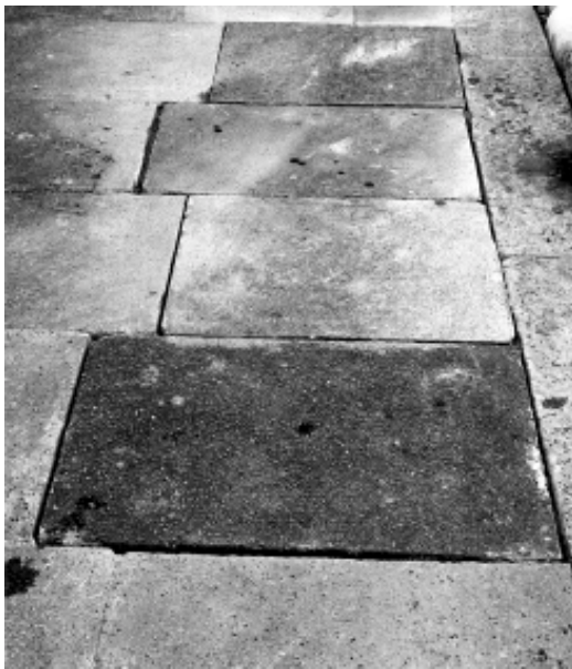
Plate 7 Absence of jointing sand between flags
