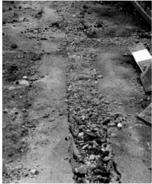
Plate 3 Poorly graded material
