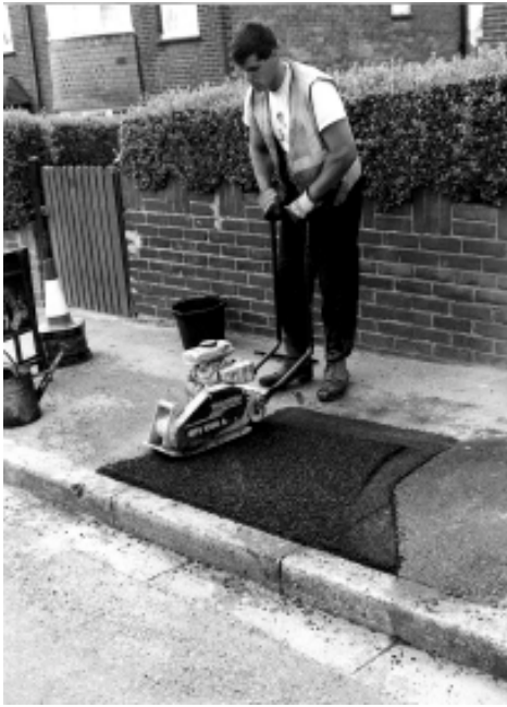
Plate 6 Unsuitable compaction plant
