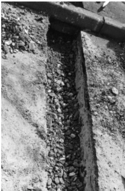
Plate 2 Poorly compacted Type 1 sub-base material
