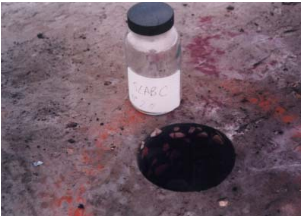
Plate 6 Carbonation of material C slab surface
