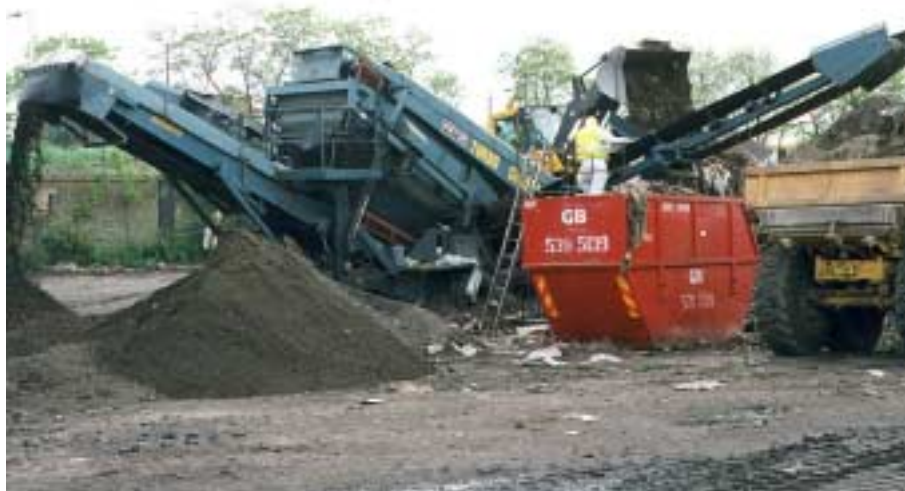
Plate 3 Mechanical sorting of old landfill material for use as Class 1A fill
