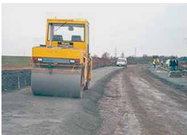
Figure A2 Placing GFA on the Burntwood By Pass, Staffordshire (Photographs courtesy of Staffordshire County Council)
