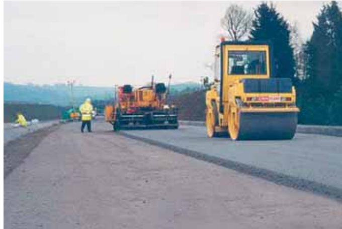
Figure A5 The use of SBM in the construction of the A485 link road, Carmarthen
