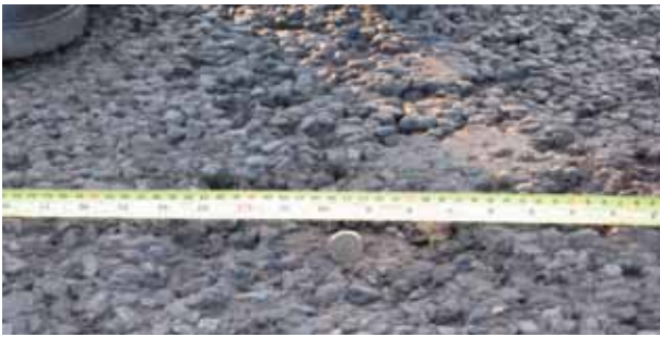
Figure 3.3 Surfacing showing excessive material loss (Site TSMA33)
