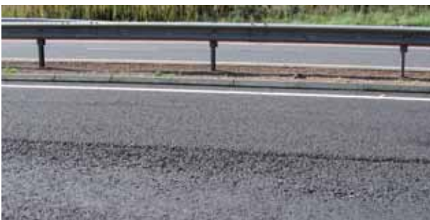
Figure 3.5 Fretting of surface (Site TAC4)
