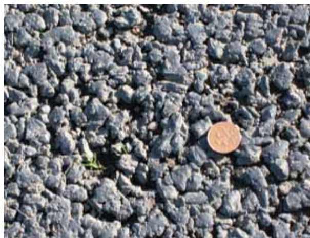
Figure 3.2 Surfacing deficient in fine aggregate (Site TAC8)
