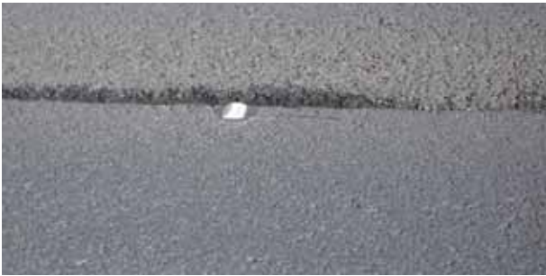
Figure 3.11 Fretting of joint at Site TAC4 (five years)
