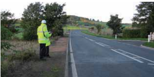
Figure 3.6 Discrete area of low texture depth (Site TAC6)
