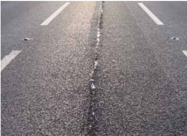
Figure 3.12 Poor joint construction at Site TAC9 (one year)
