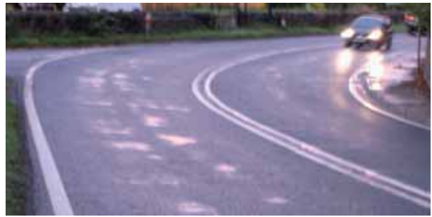
Figure 3.7 General flushing of material (Site TSMA11)
