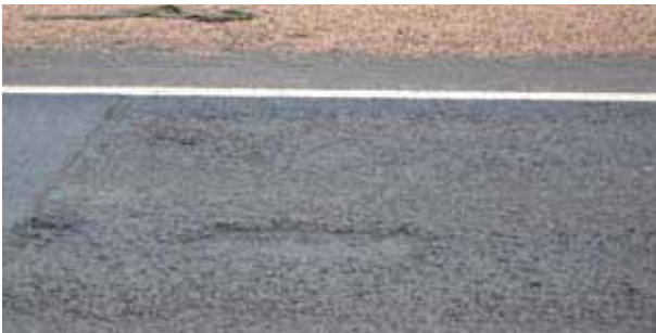
Figure 3.4 Fretting of surface (Site TAC3)
