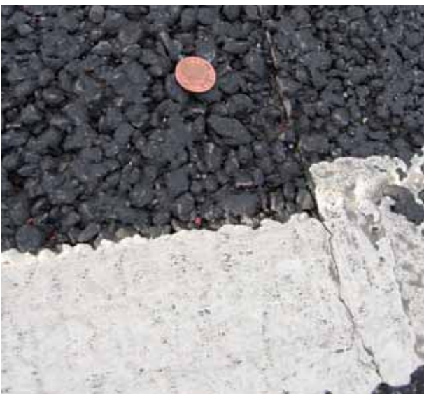
Figure 3.13 Sawn joint not sealed at Site TAC9 (one year)
